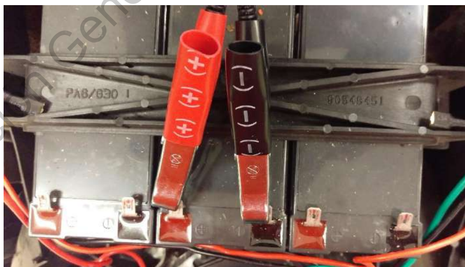
Figure 63. Clamps attached to battery terminals.
